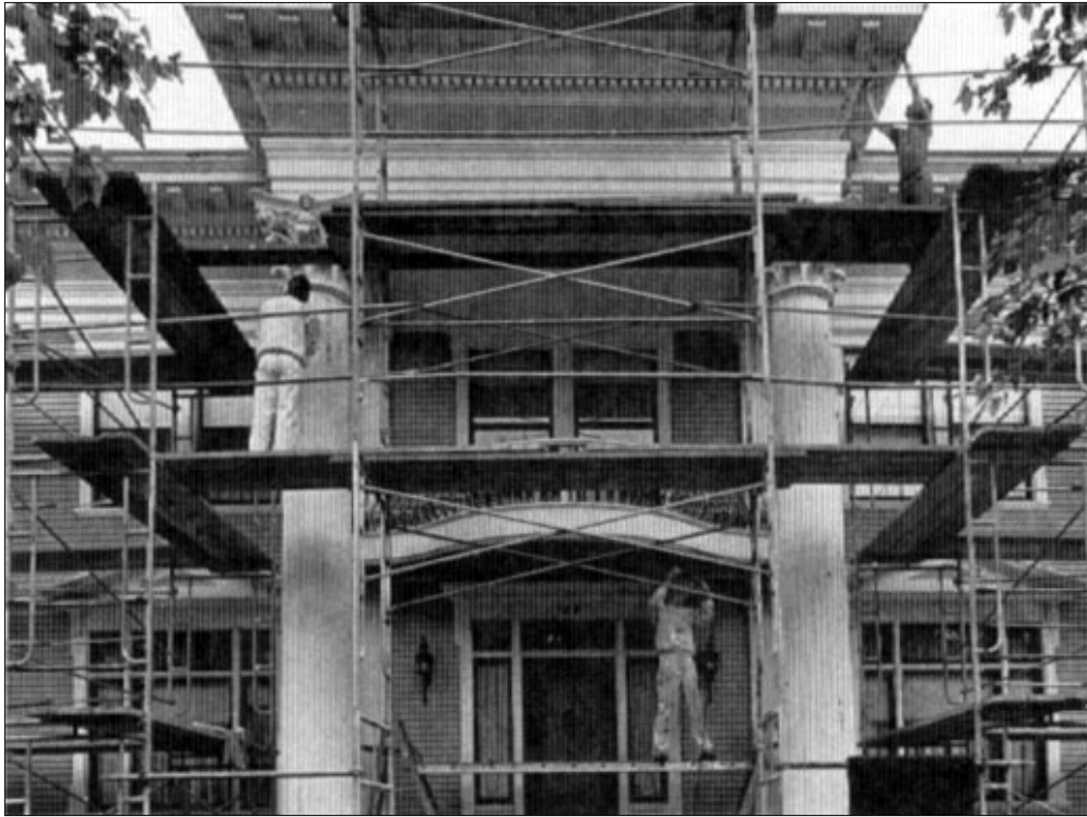
Ongoing work at this house focuses on the maintenance and repair of exterior wood features from the restoration period. After scraping and sanding, the wood was painted in colors documented to the Restoration period. Photo: ©Mary Randlett, 1992.
